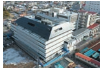
New Main Government Office Building, Ueda City (air conditioning and plumbing works)
