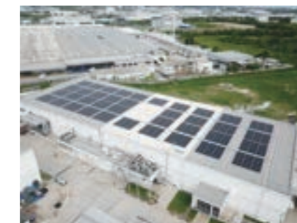
Thailand Solar cells for existing factory (Company P)
