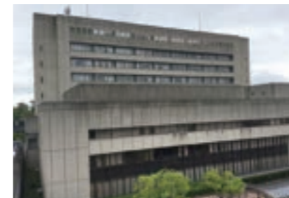
Major renovations at government office building, Tsu City (electrical, air conditioning and plumbing works)
