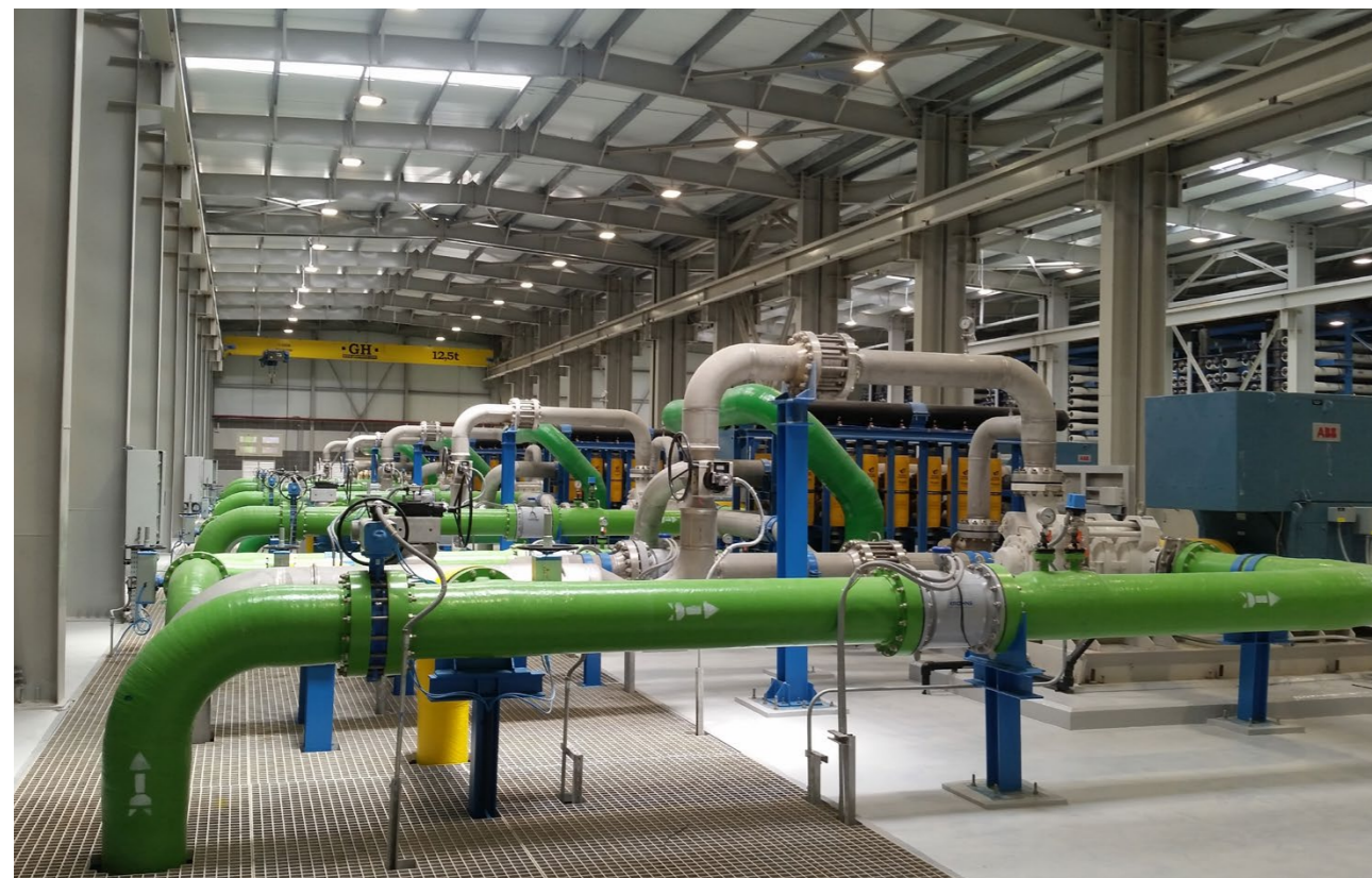
Sea Water Desalination Plant (SWDP) in Mostaganem, Algeria.
