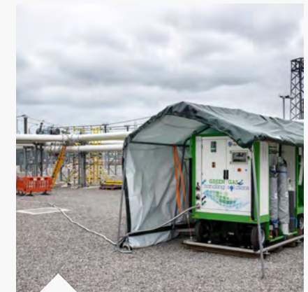
Onsite gas cart used to retrofill existing Gas Insulated Busbar with an alternative low global warming g3 gas designed for high-voltage transmission equipment
