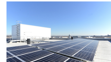
Solar Panels at ANA Blue Base
