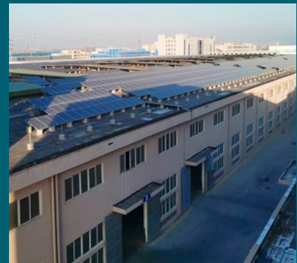
Solar panels on top of the production plant in Shandong.
