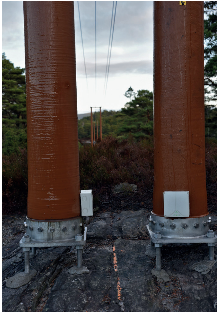
A new foundation system for composite utility poles on bedrock has a significantly smaller footprint than other traditional methods.
