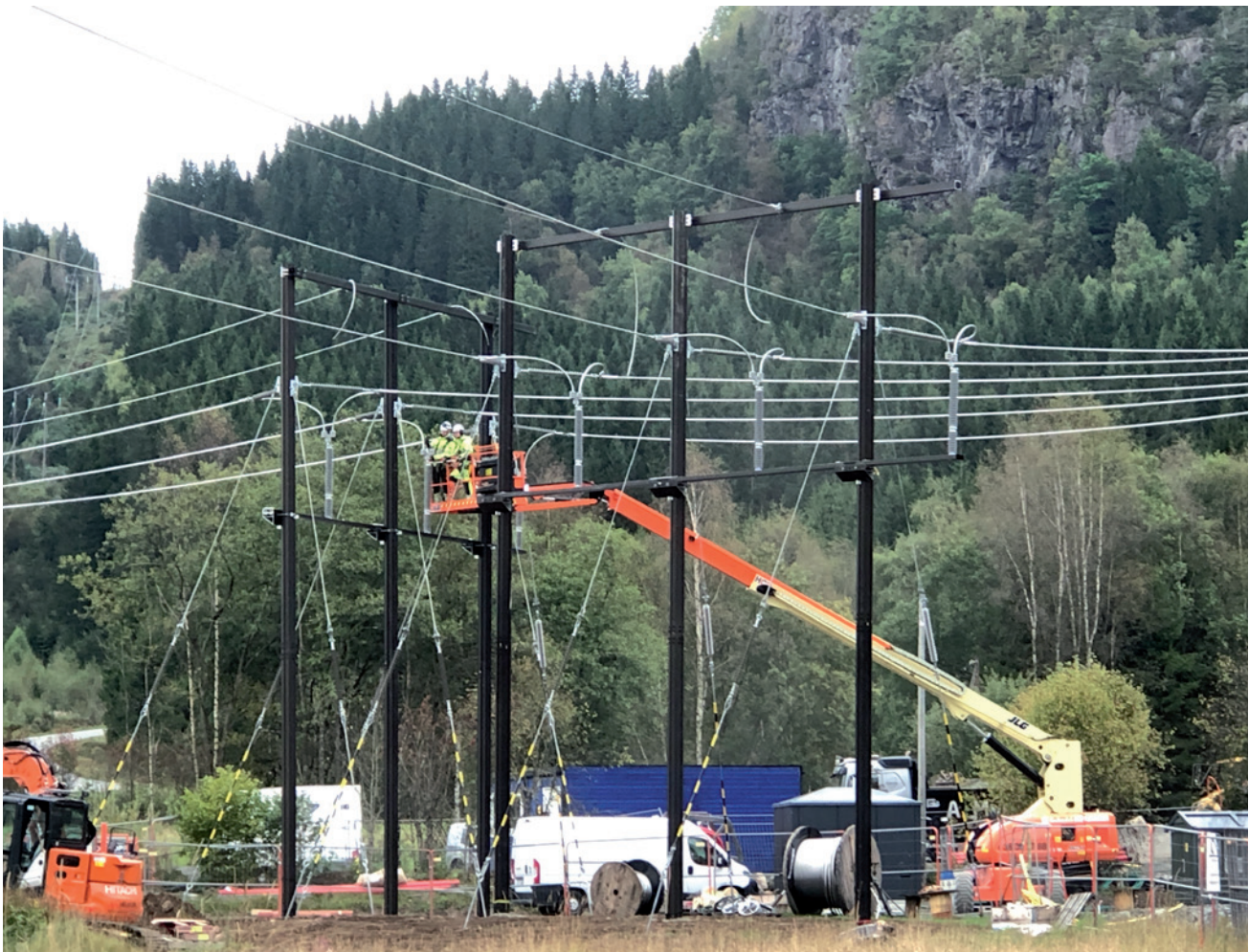
Agder Energi Nett is testing alternatives to creosote utility poles, which are not ideal from an environmental point of view. At Austerdalen substation in Kvinesdal poles made of aluminium are installed. The substation, which was commissioned in 2021, was built to allow the grid to cope with more renewable electricity.
