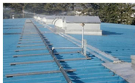
Running status of circulating roof spray system
