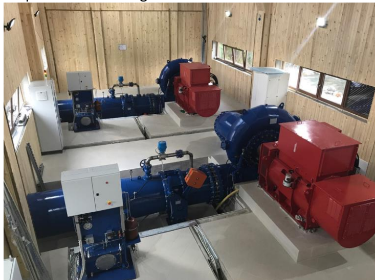
Hydropower plant developed with Vaptech technology and systems
