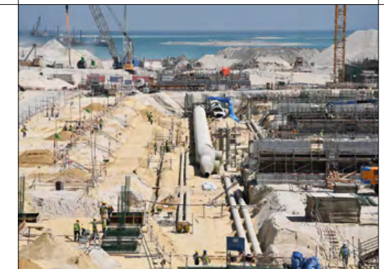
Jubail desalination plant, Saudi Arabia
