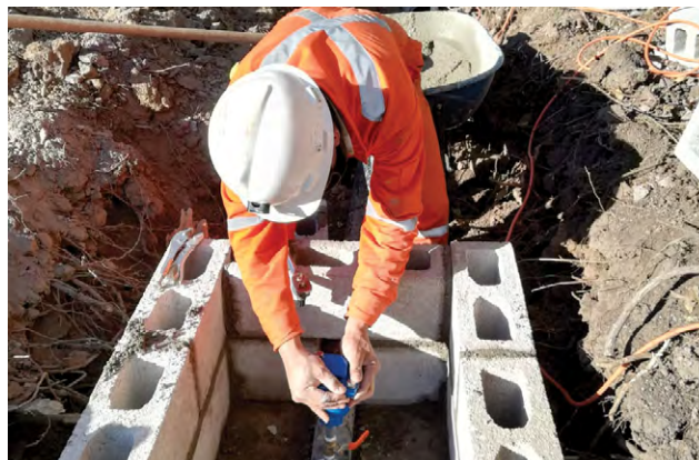
Guazapares water filtration installation
