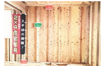
Example of construction of wall frames using Japan-grown timber (Ichikawa Home Gallery)
