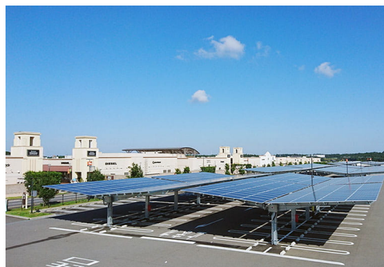
Shisui Premium Outlet's carport-type solar power generator for captive consumption
