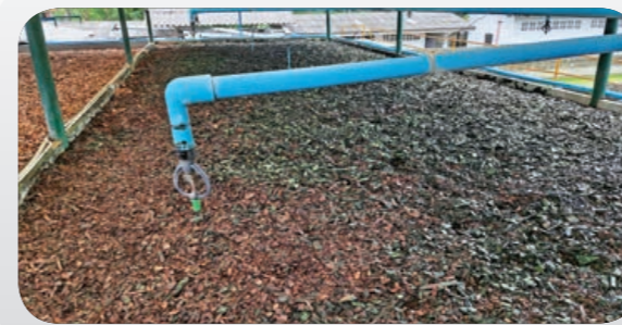
Biofiltration system at Thungsong factory, Teck Bee Hang in Thailand.
