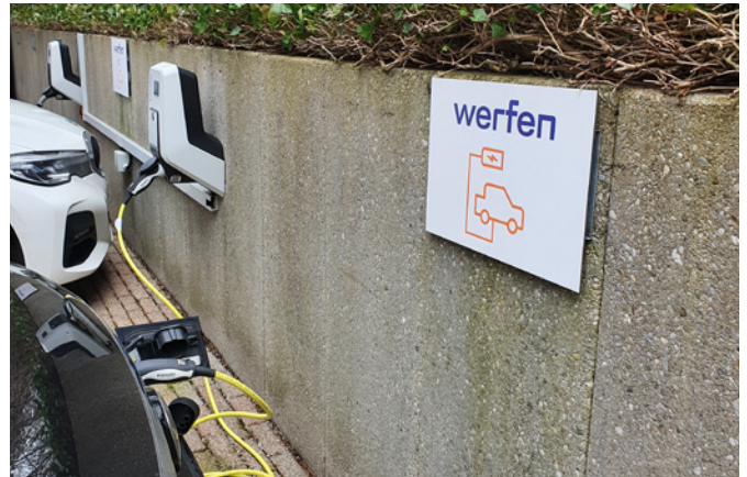
One of the charging stations in Munich in action.
