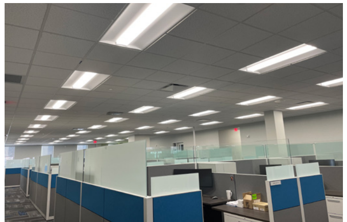
LED bulbs were installed in the Bedford, MA, facility in the US.
