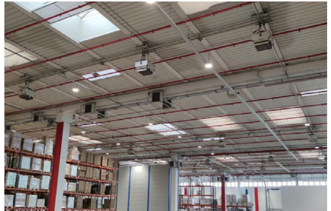
LED bulbs were installed in our Roncello facility in Italy.
