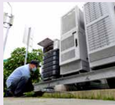
StarHub Mobile Base Station
