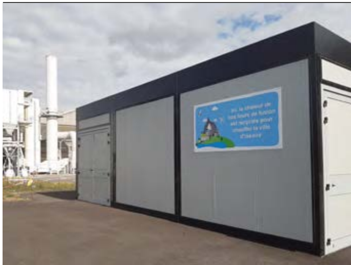
▲ This building contains the heat exchanger that provides heat to the city of Issoire
