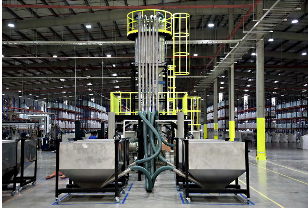
Nike Air Manufacturing Innovation Facility – Dong Nai, Vietnam
