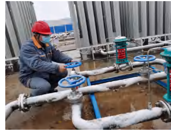
▲ Adjust the pressure of the air supply system for Leishenshan Hospital to ensure the stable oxygen supply of the ventilator
