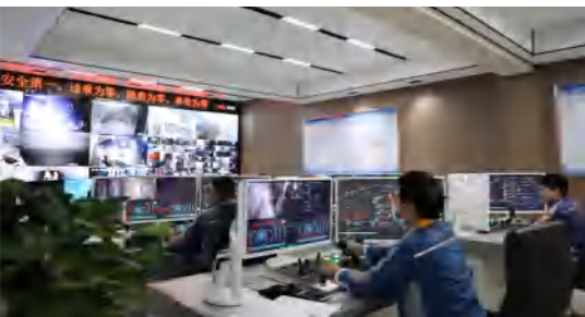
▲ Operate downhole instruments in the central control room
