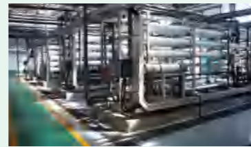
▲ Coking waste water treatment
