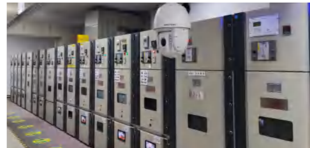
▲ Remote intelligent inspection robots of centralized power control system
