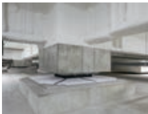
Seismic isolation rubber and seismic isolation dampers (Misato Distribution Center No. 2 Phase 2 building, Tokyo)
