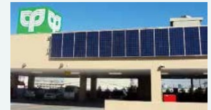
Solar panels installed on building walls
