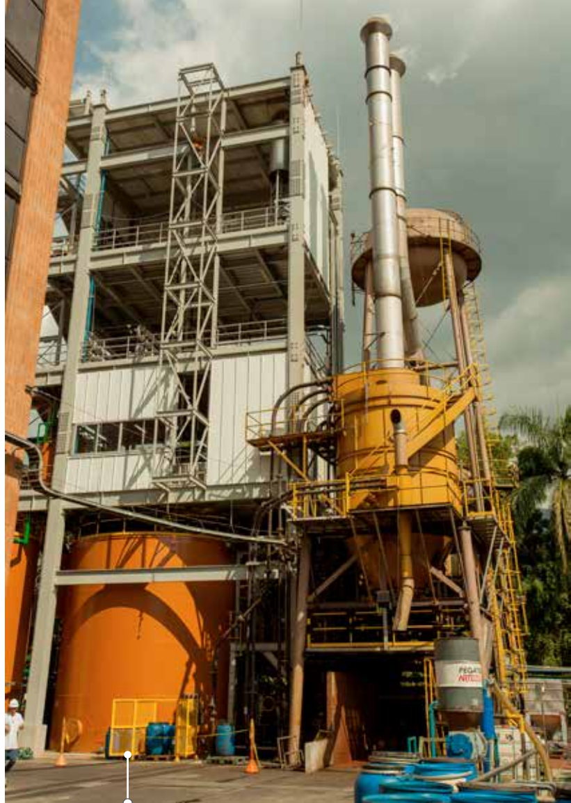
Wastewater treatment plant at the Coffee Business in Medellín, Colombia.
