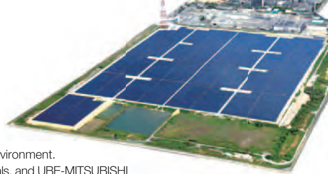
Solar power plant
