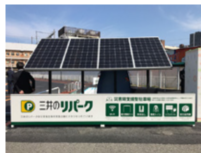
Solar power panels of the hybrid solar system at the Mitsui Repark Minatomachi Niigata Parking Lot
