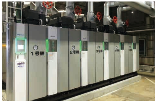
Fuel equipment at Toyama Daiichi Plant
