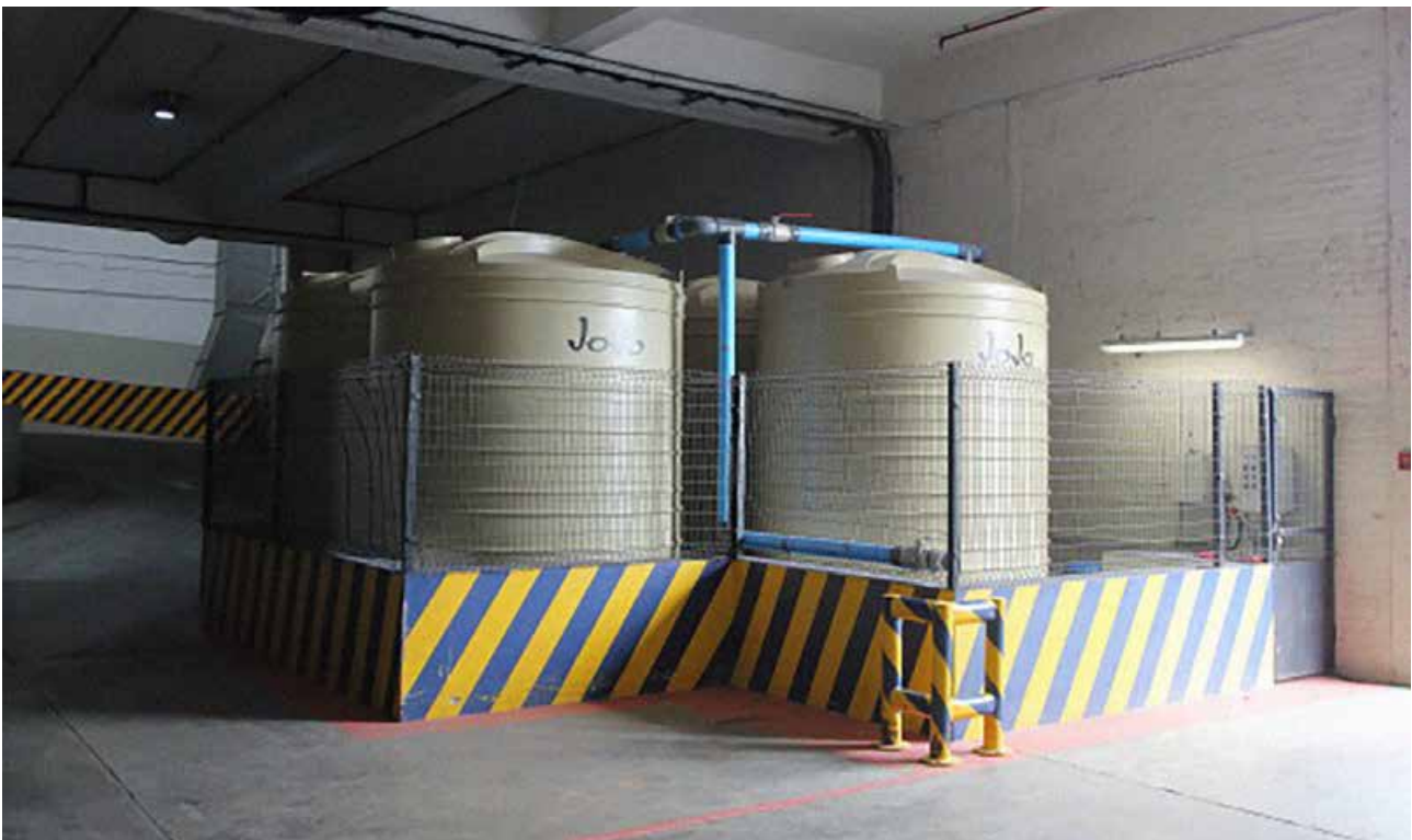
Rain water harvesting and borehole water tanks at the head office.
