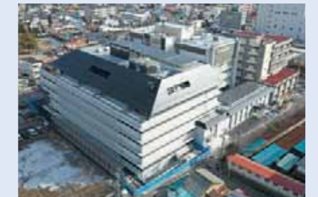
New Main Government Office Building, Ueda City (air conditioning and plumbing installations)
