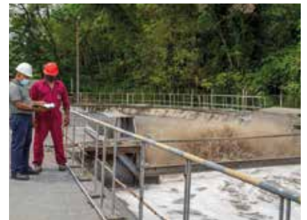
Modern effluent treatment plant ZDHC compliant since 2017
