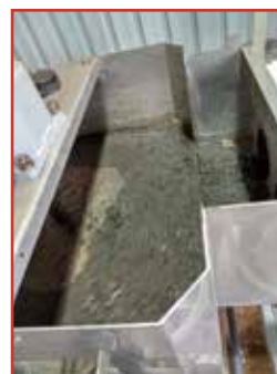
Sludge Mixing Tank
