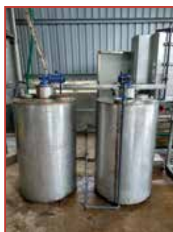
Chemical Mixing and Dosing Unit
