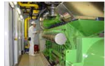
Cogeneration system at Tonegawa Brewery
