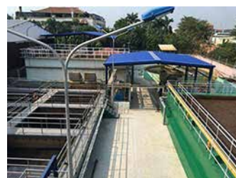
Waste water treatment plant
