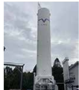
Once-through Boilers and LNG facility at OSUMISYUZO LIMITED
