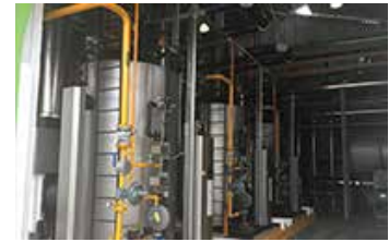
Newly installed once-through boilers at the Beam Suntory Sauza Plant in Mexico
