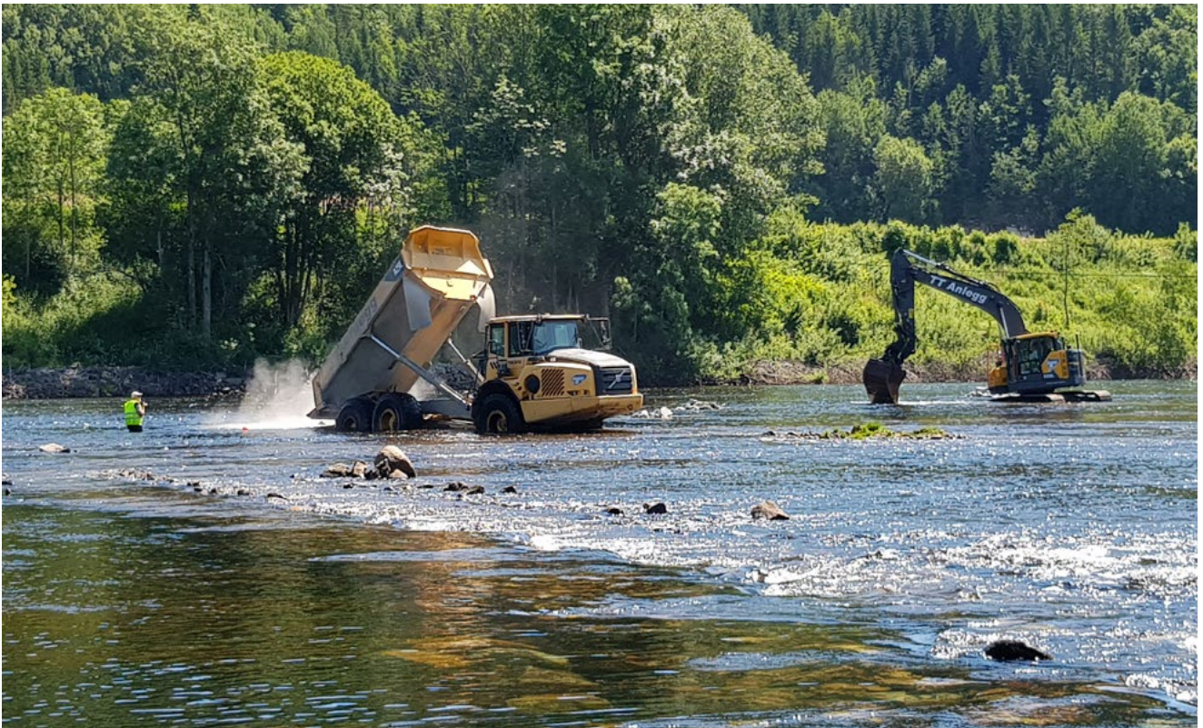
Agder Energi has been working to develop a large nursery for young salmon at Froland on the River Nidelva. Here stone blocks are put out at suitable locations in the river, which creates good hiding places for the juvenile salmon.
