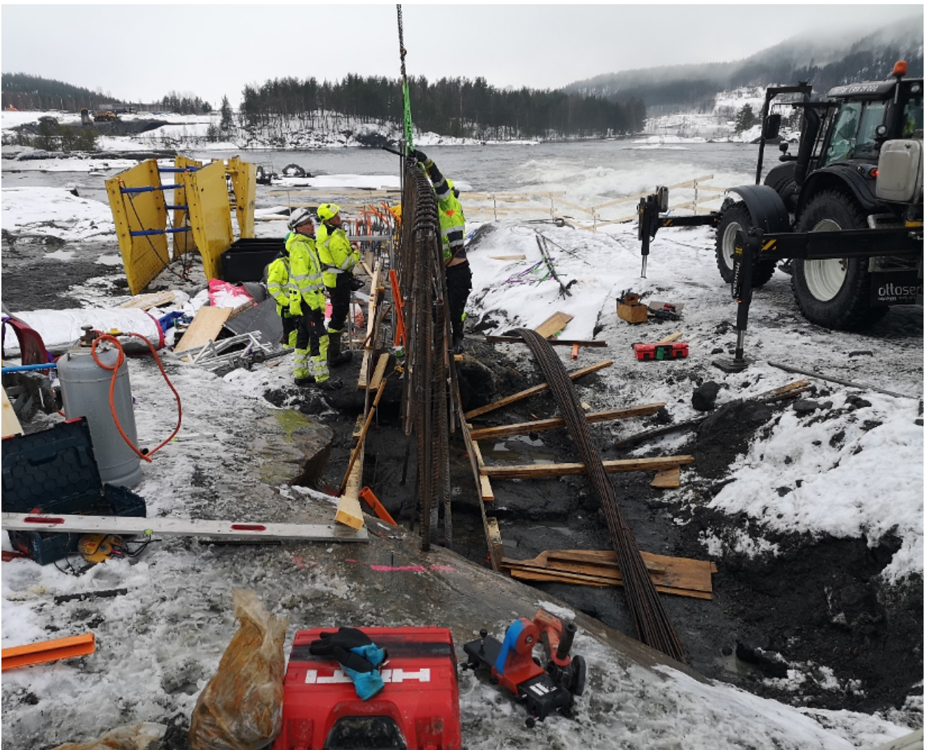
Each year, Agder Energi spends large amounts of money on buying goods and services; here work on Fennefoss power station in Evje is well underway.
