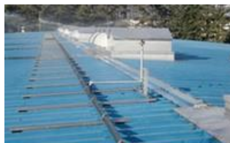
Running status of circulating roof spray system
