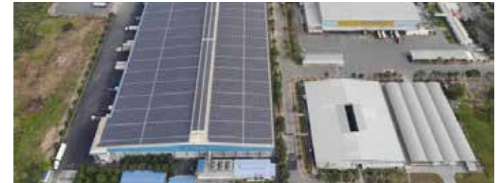
CJ GMD Logistics Center Solar Power Facility
