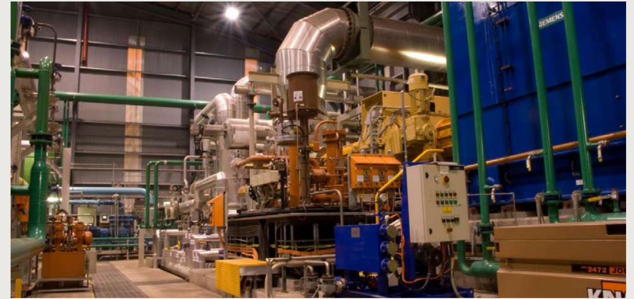
Steam turbine-generator room at our Australia sugar mill
