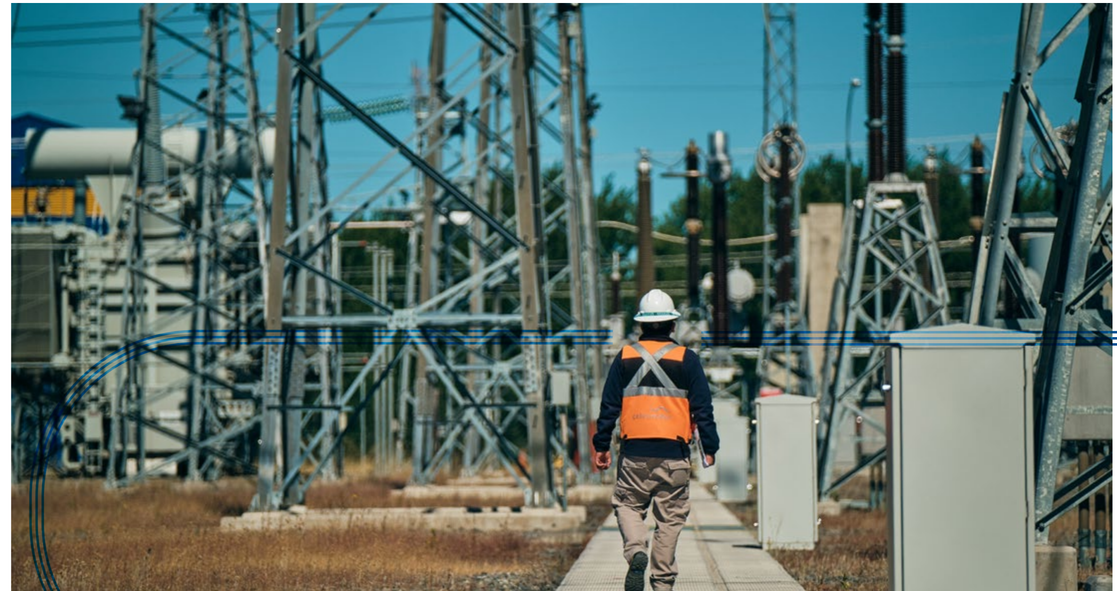
SUBSTATION CHARRÚA (CHILE)
