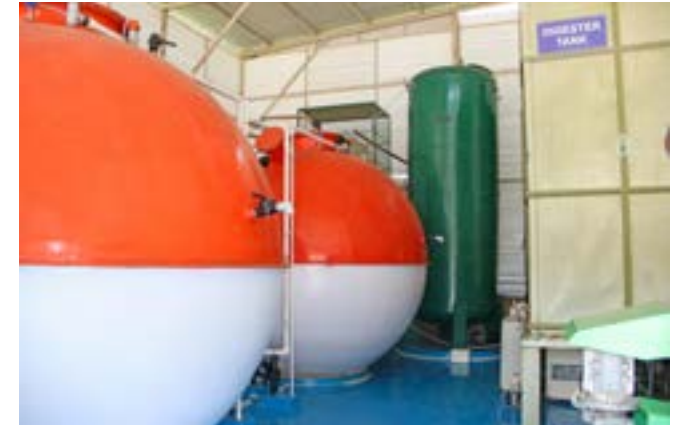
Biogas plant at an Infosys campus
