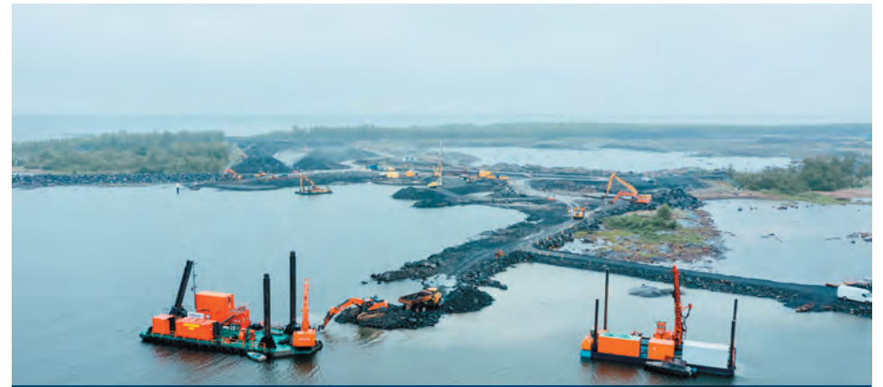
In the sea area, the RAOS Project continued with the water construction work and dredging of the nuclear power plant's cooling water discharge channel, the cooling water intake structures, and the construction work of the harbor.
