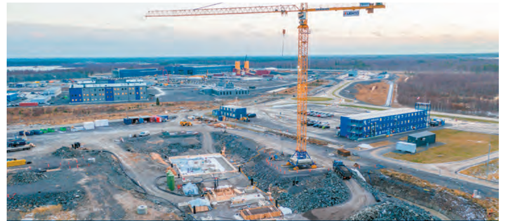
Lehto Group began the construction of Fennovoima's administration building in August 2020. The administration building is planned to be completed at the first half of 2022.
