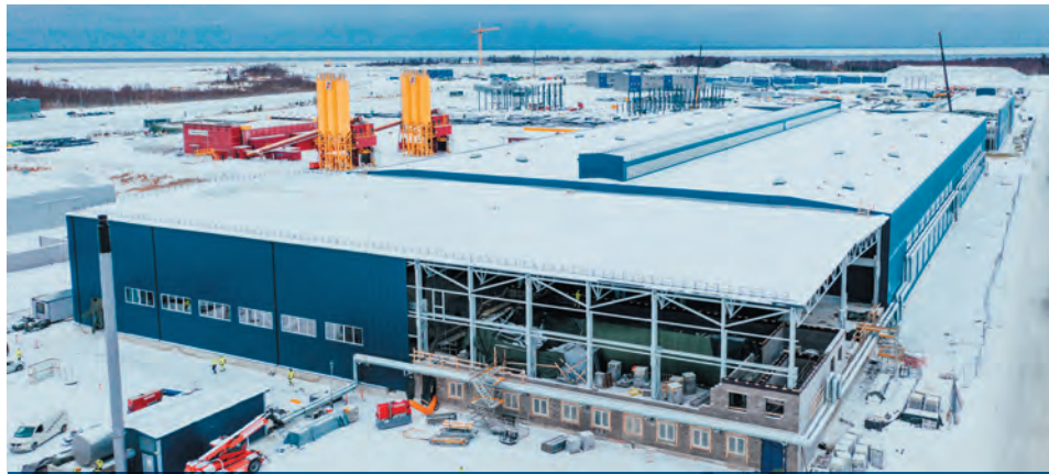
In the plant supplier's support functions area, construction work on the reinforcement workshop and the anticorrosion treatment workshop continued. In addition, the plant supplier began the construction of storage areas and workshops, which will be used for the storage of plant components.
