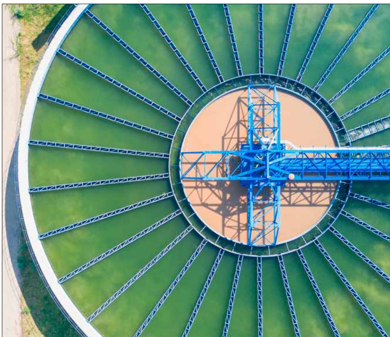
Water treatment plant made with stainless steel components
