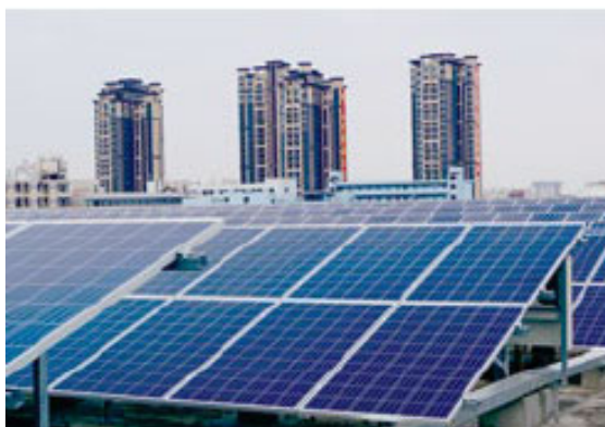
Solar power panels installed on the roof
