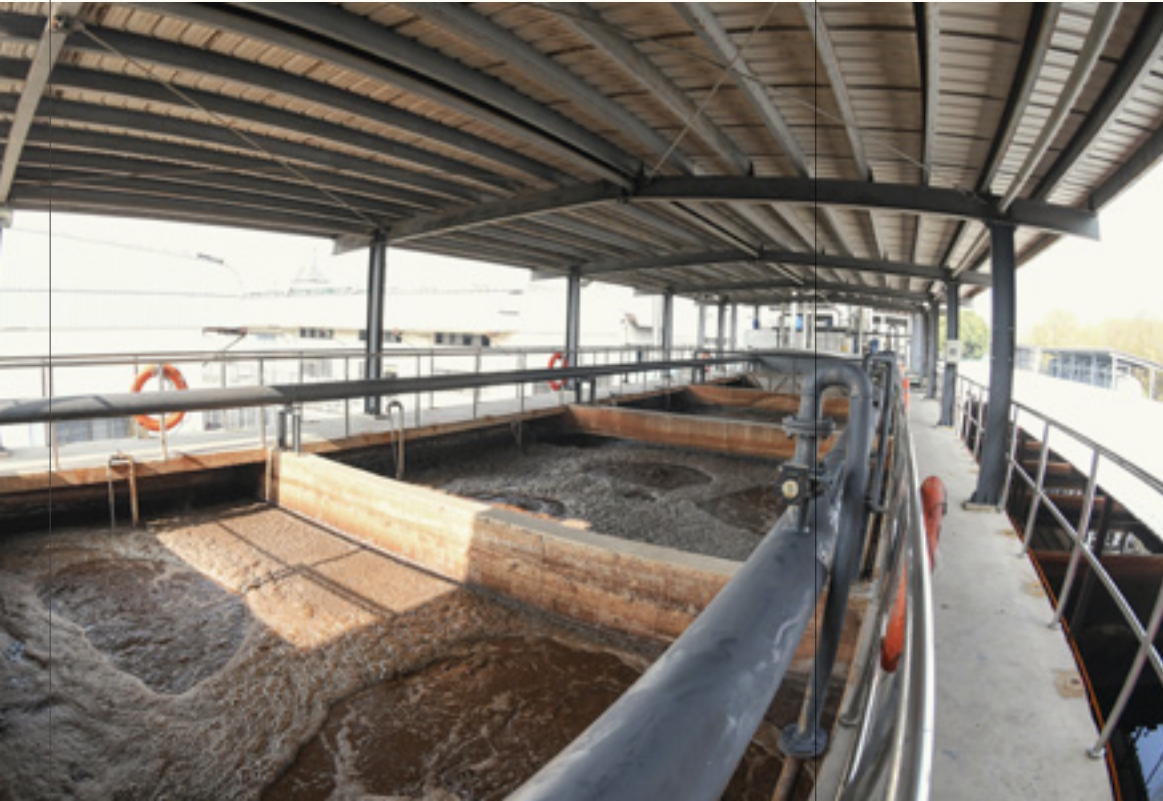
State-of-the-art wastewater treatment at the Ramatex textile mill in Suzhou, China
