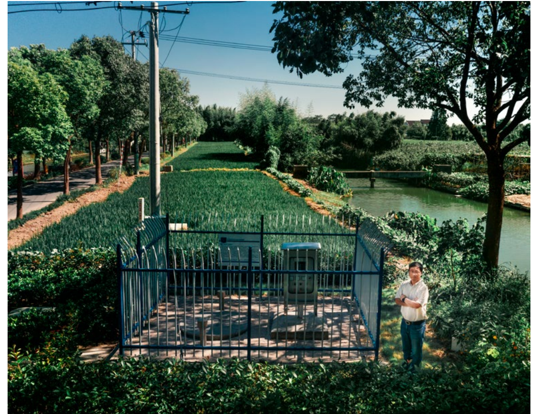
China Business Network (CBN) acknowledged our work in China, and awarded Grundfos China with CSR Environmental Ecological Contribution Award 2020. Read our wastewater solutions in Pudong, China on page 18
