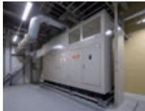
Emergency power generator (Minamihonmoku Distribution Center in Yokohama)
