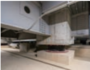
Seismic isolation rubber and seismic isolation dampers (Ibaraki Distribution Center No. 4 in Osaka)
