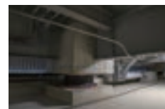
Seismic isolation equipment
