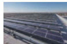
Solar power generation equipment
