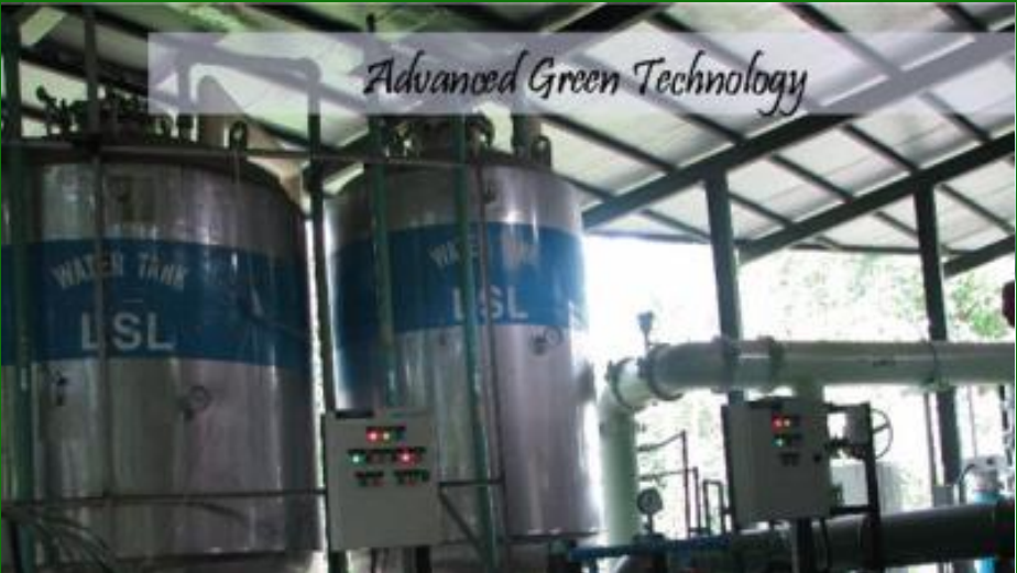
4 th Generation Heat Exchange Chiller System recovered heat waste is used for the hot water supply and hot water spa pool
