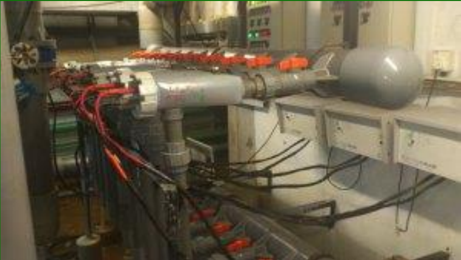
Swimming pool ionization treatment systems
