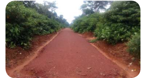
Secondary road built in January 2019, abandoned 8 months ago.
