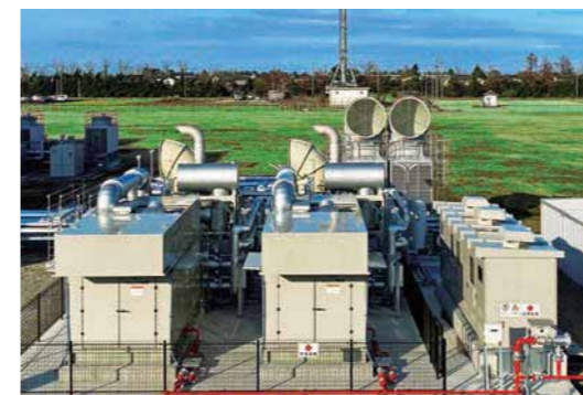
Cogeneration System Facility, Toyama Factory Otsuka Pharmaceutical Factory, Inc. (electrical and air conditioning installations)
