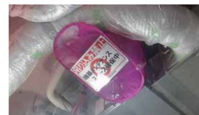
Makes visible the maintenance point of ceiling-embedded equipment during the construction period.
