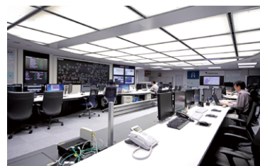
Supply Control Center
