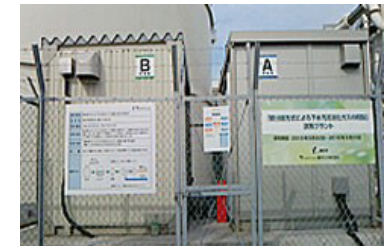
Biogas refining test equipment installed at North Yokohama Sludge Recycling Center
