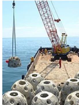
Installing artificial reef balls Source: Petronas, "Bringing life to a barren ocean"
