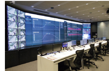
Central monitoring room in the Nihonbashi Energy Center
