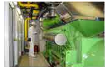
Cogeneration system at Tonegawa Brewery
