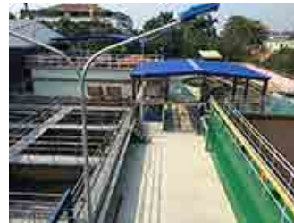
Waste water treatment plant
