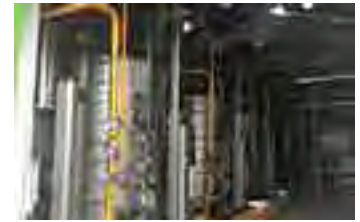
Newly installed once-through boilers at the Beam Suntory Sauza Plant in Mexico
