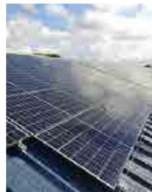
New solar panels installed on the roofs of the fermentation facility
