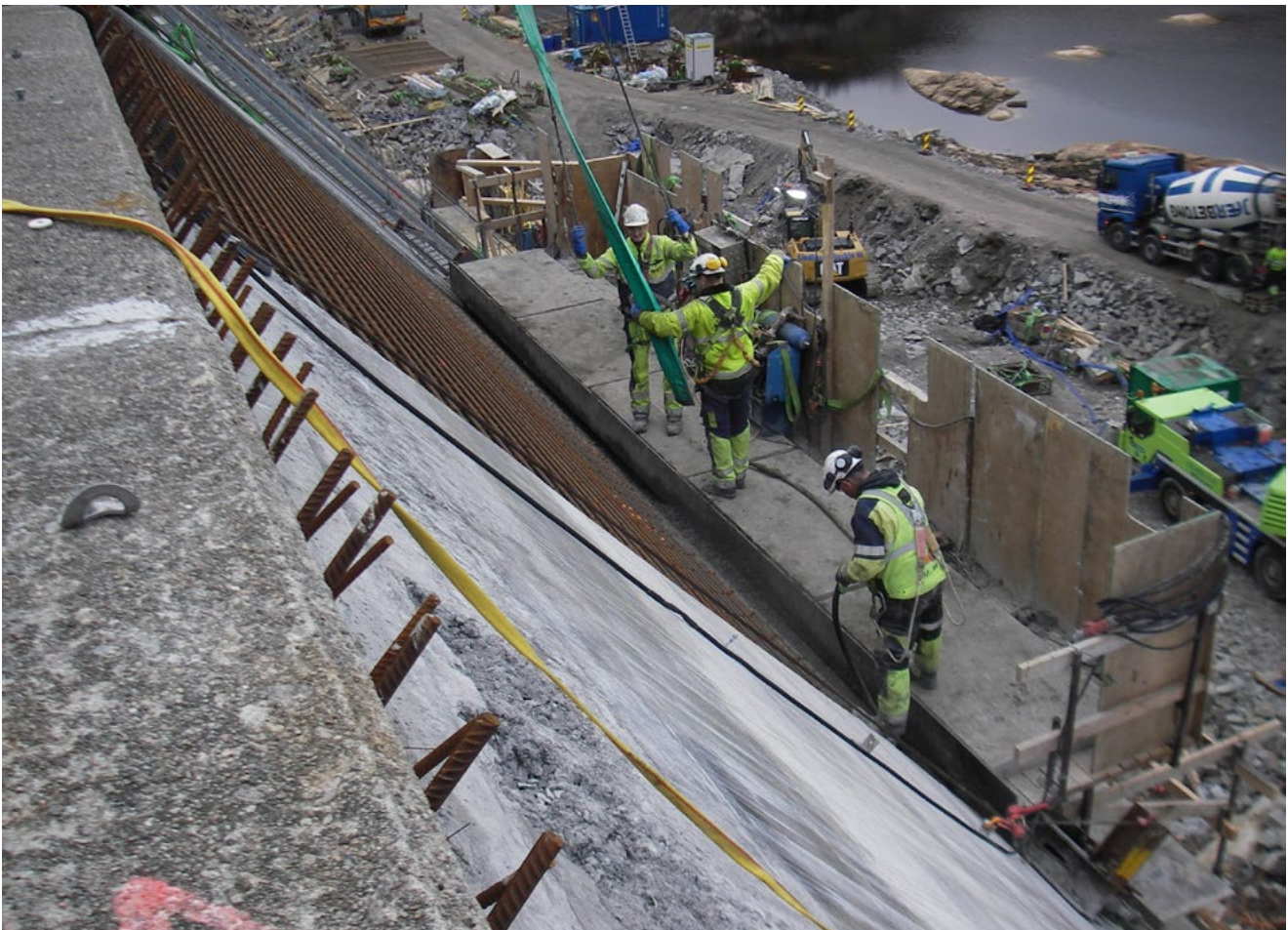
Each year, Agder Energi spends large amounts of money on buying goods and services. Here work is being done on Kuli dam in Sirdal.
