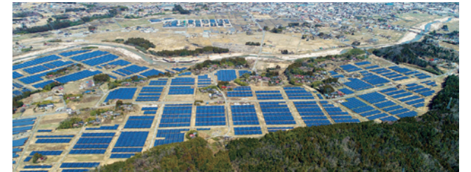
Namie Sakai Solar Power Plant 1 and 2 in Namie Town, Fukushima Prefecture, Japan
