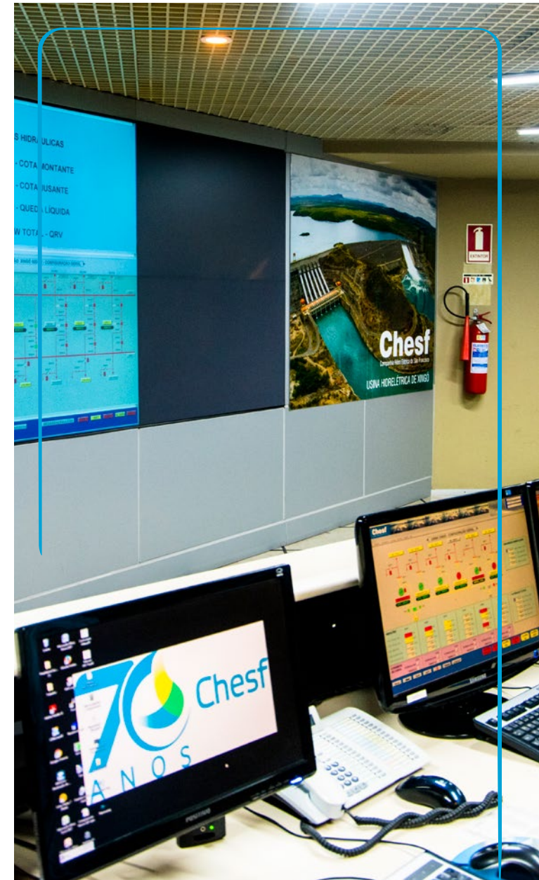
Command center at the Xingó plant in Sergipe. Credit: André Schuler.
