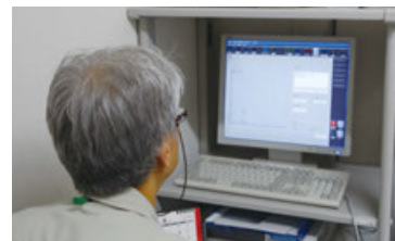
Demand monitoring equipment at the head office building
