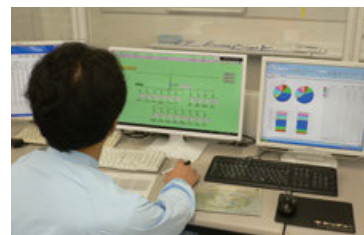
Power monitoring system of the Fukusaki Factory
