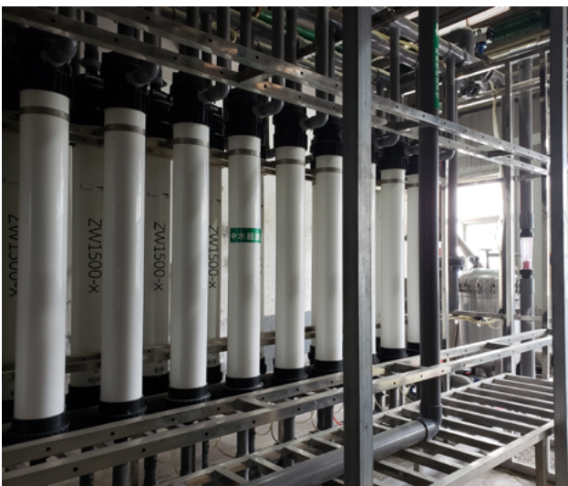
LONGi Xi'an Slicing Factory Sewage Treatment Station
